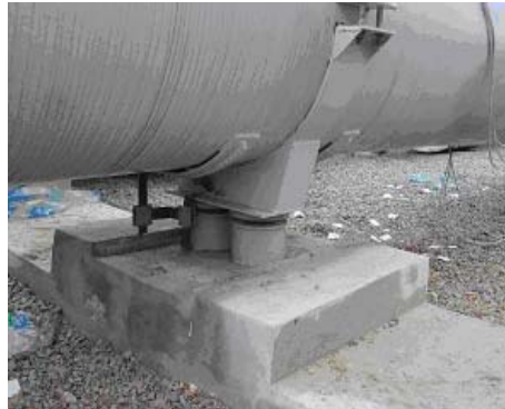
Figure 9. Supporting foot of pipe with metallic dampers
