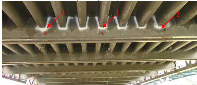
Fig.2 AE sensors position on places 0, 1, 2 – 32th span
