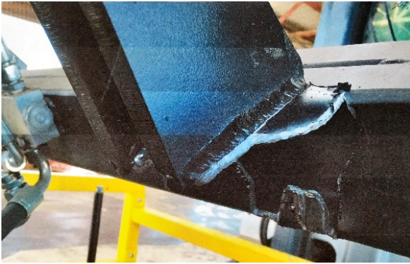
Fig. 2: Damage of the console for the hydraulic cylinders.
