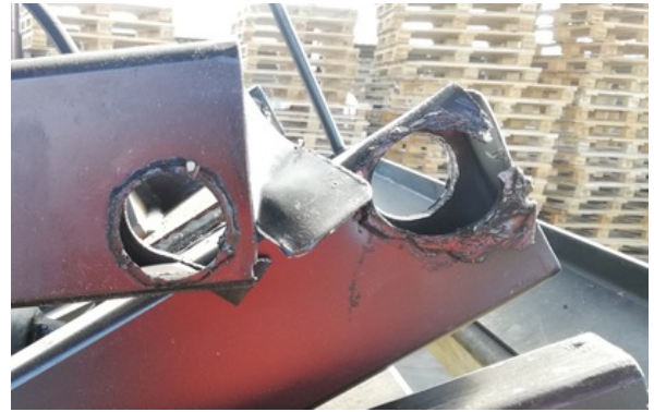
Fig. 3: Damage of the pin joint.
